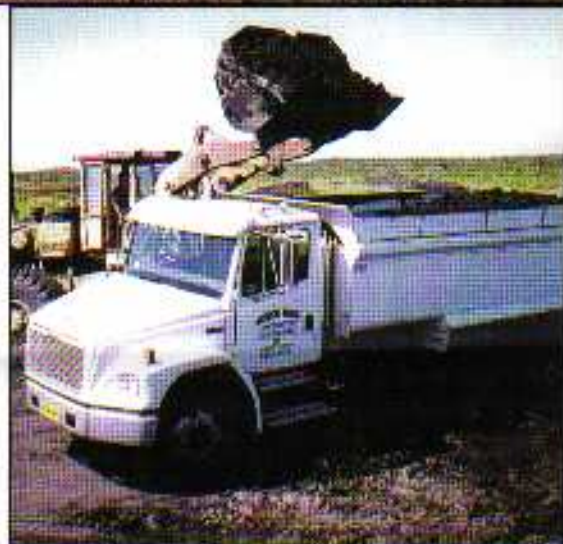
Top: Conventional mud/ash spreading (works well in dry weather). Below: wet weather conditions necessitate reloading from stockpiles.
